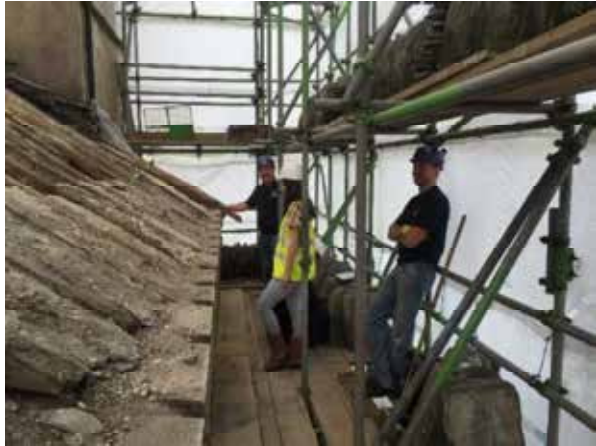
Carrying out an inspection of the roof with main contractors and directors of HCR, Mick and James
