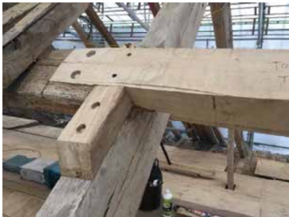
Completed purlin repair. Stainless steel fixings were used and a new oak block installed to give the purlin additional support
