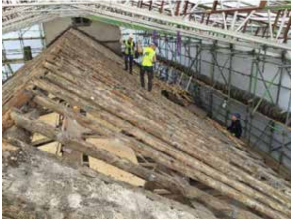
Slates being carefully removed and stacked in order, any replacement slates were slotted in at the appropriate place to ensure slates that were remaining went back in their original position
