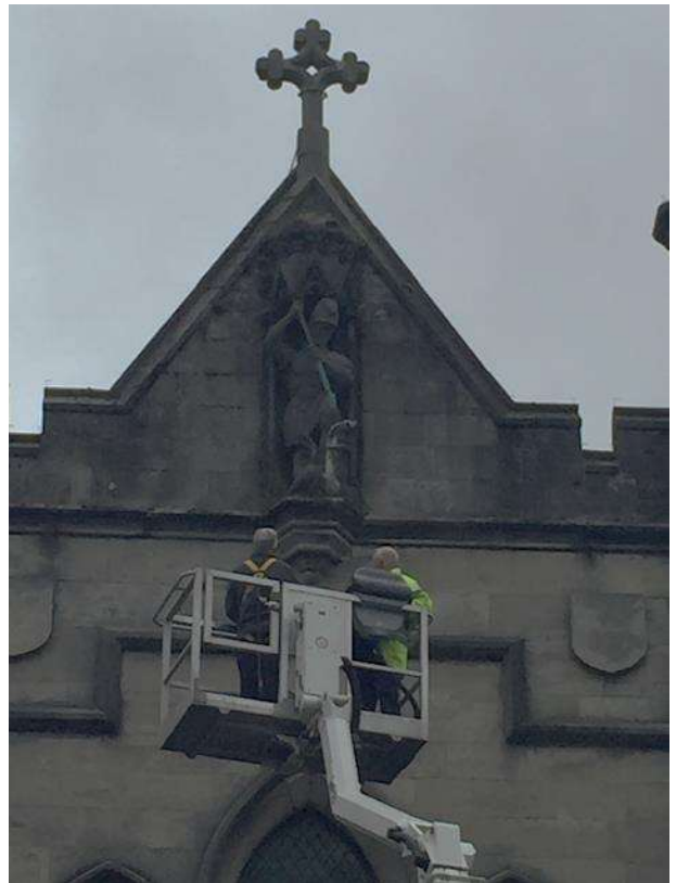
Following the survey the priest had a look at some of the defects up close to assist with understanding of the issues encountered.
